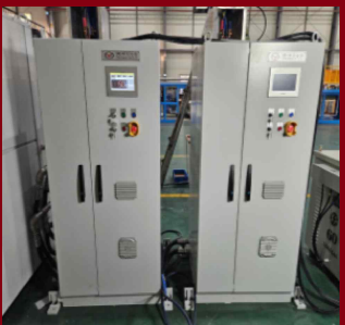
120kW+70kW Warm Forging Heater
