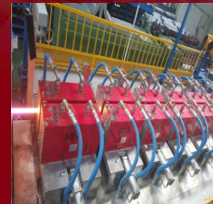
2400kW Hot Former Heater
